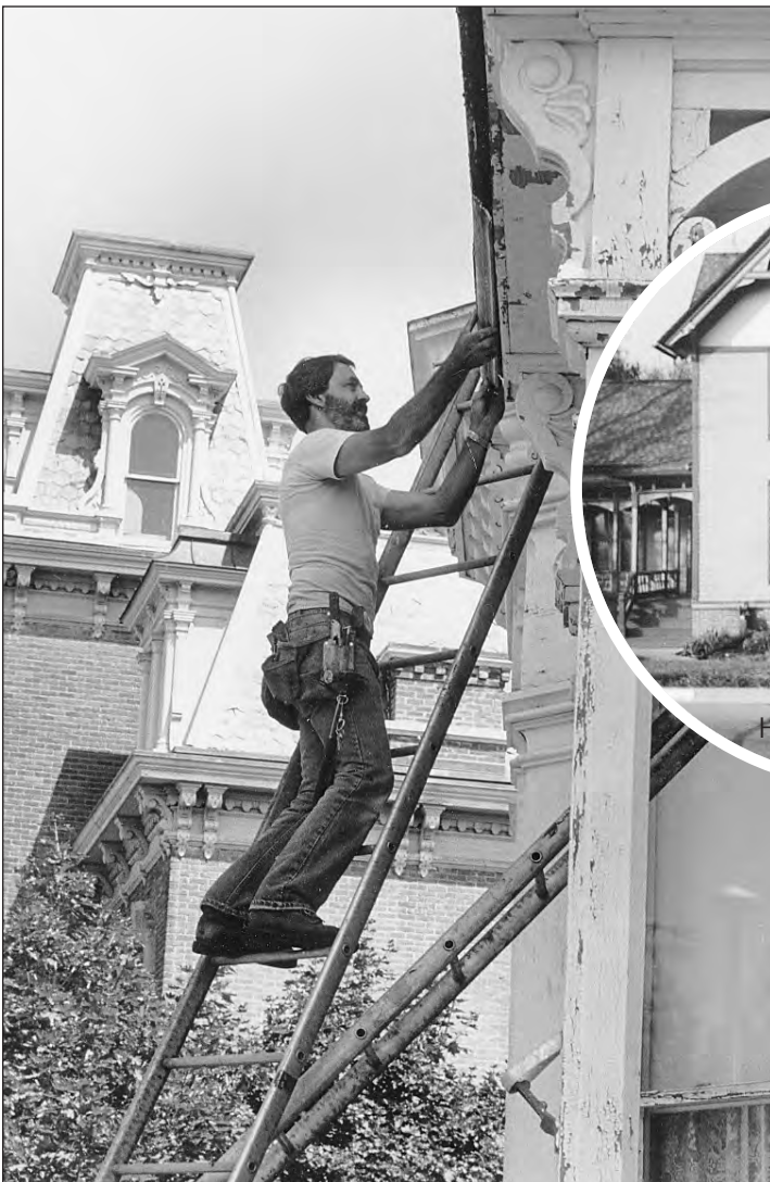
Board Member, Don Randazzo repairing the exterior of the Ypsilanti Historical Museum.
